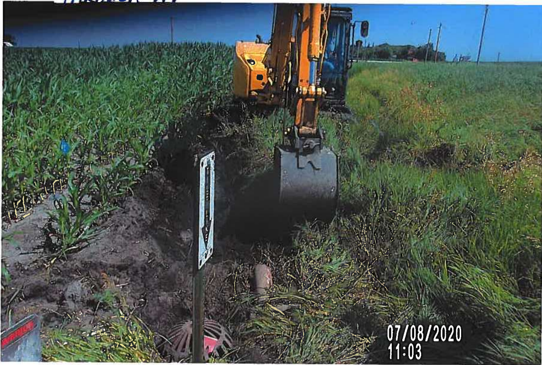
PICTURE # 4058 IS LOOKING NORTH - SHOWING CREW EXCAVATING ALONG FIELD EDGE IN WEST DITCH OF COHWYS-27 TO EXPOSE TILE TO CHECK CONDITION, FLOW AND RUN LOCATE CABLE THROUGH IT.
